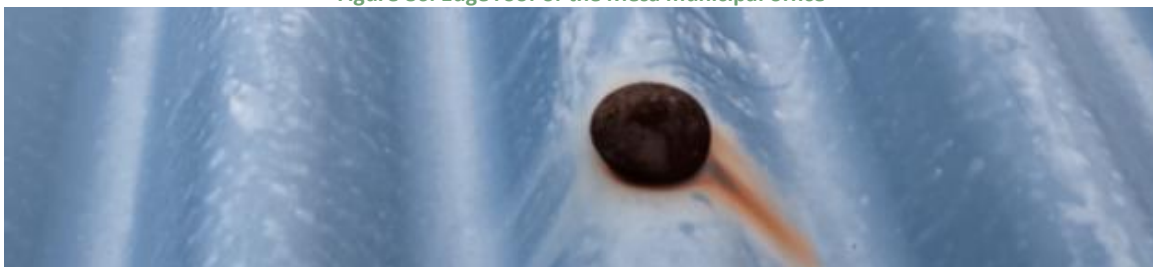
Figure 87. Rusty nails of the Mesa municipal office
