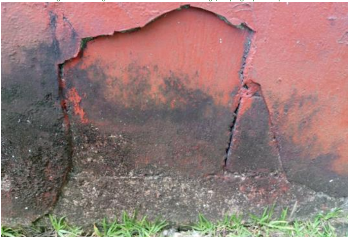
Figure 53. Footings of the Fein new church. No damage, only slightly on the plaster 2
