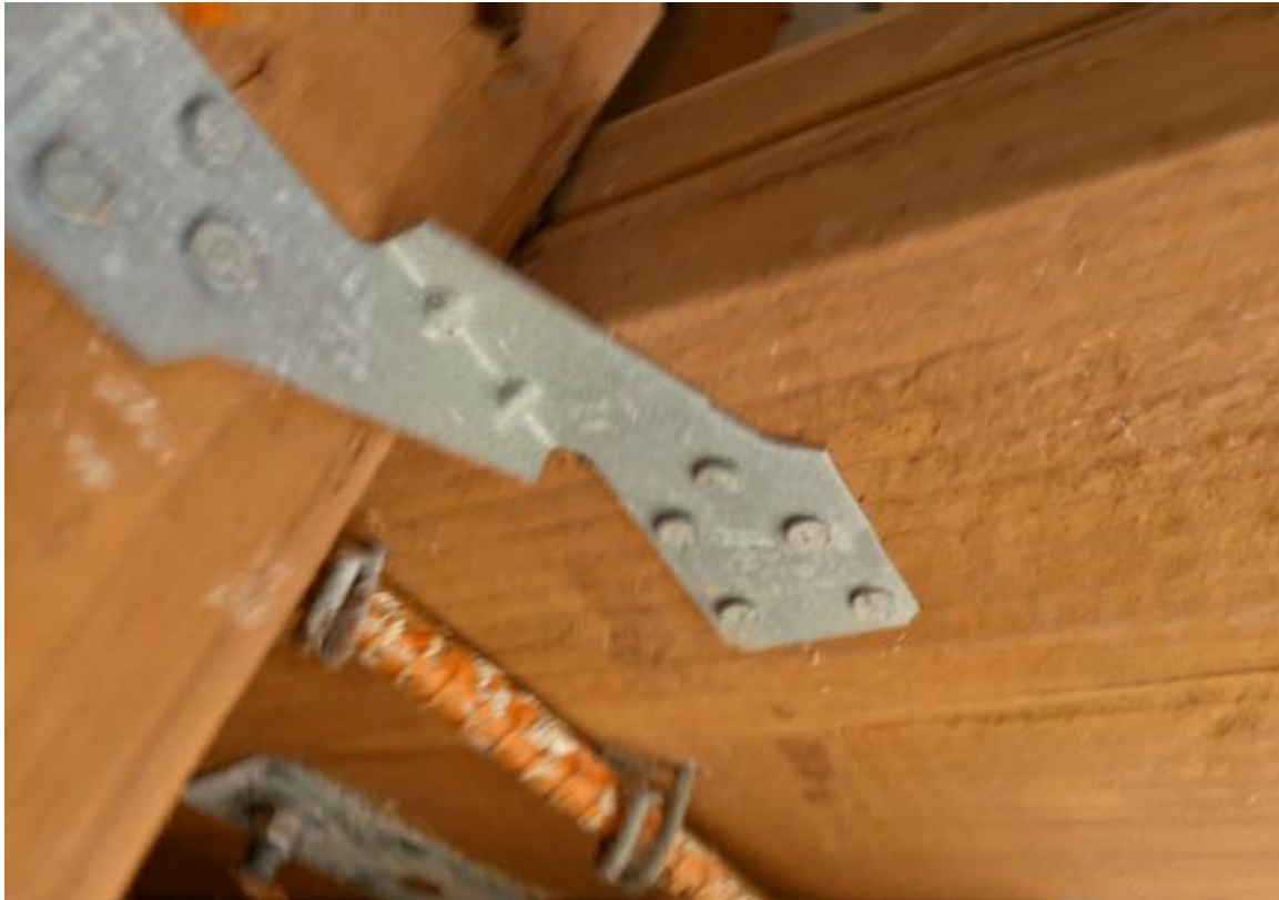
Figure 95. Mesa church rafters-structure fastening, tied to a steel bar coming out of the wall
