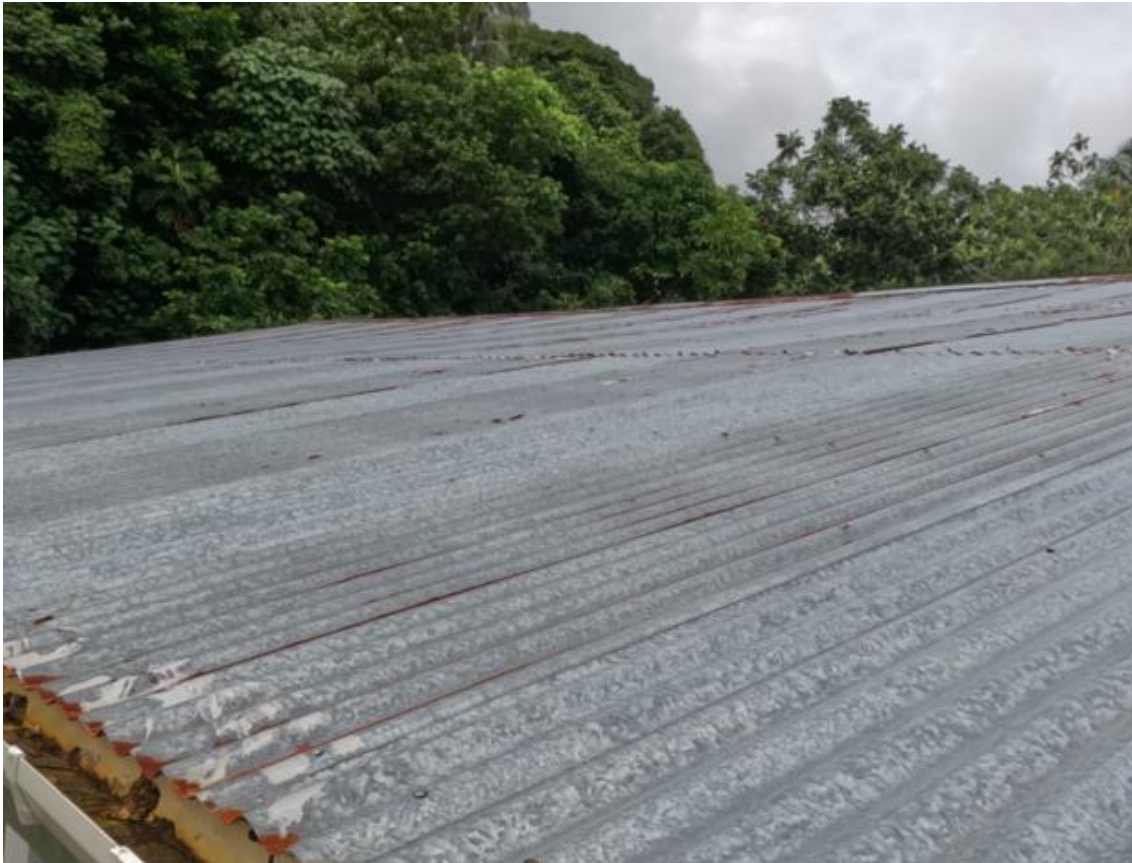
Figure 99. Western view of the Mesa church roof and trees to be trimmed by the community
