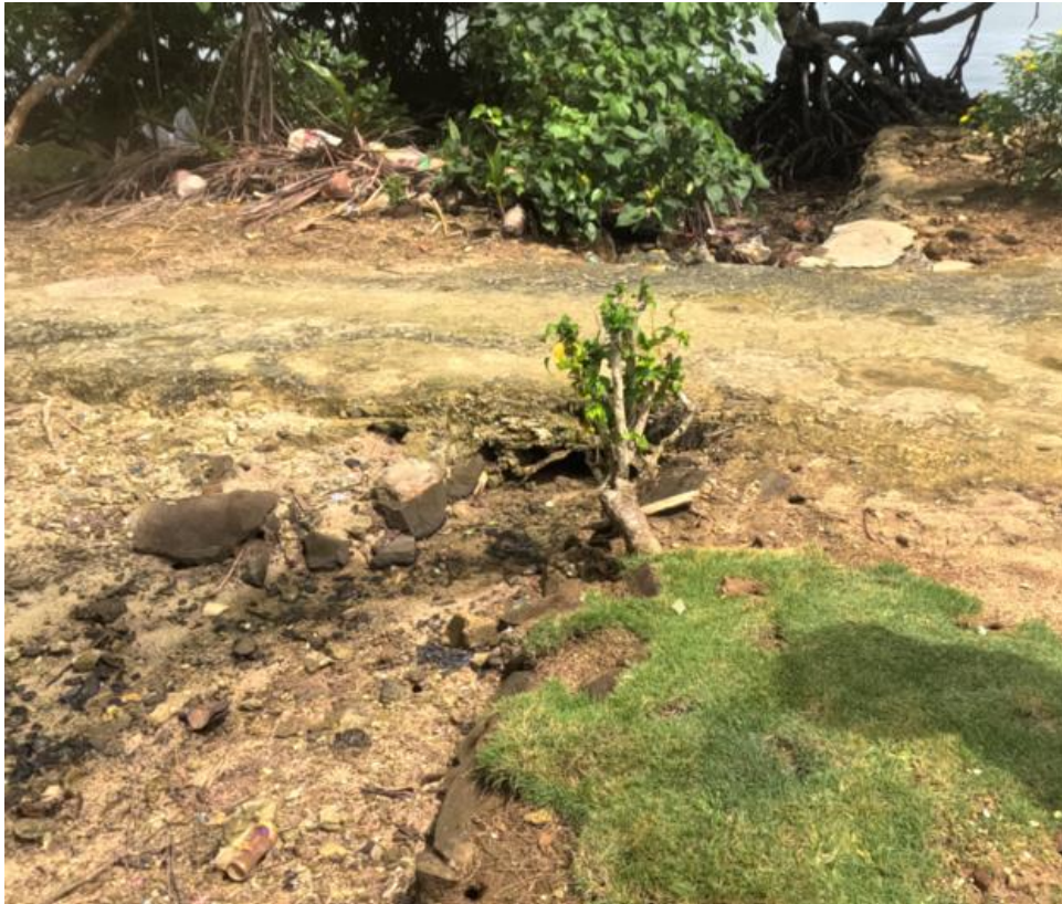
Figure 101. Mesa road and a small creek (Concrete pipe for road crossing in the middle of the picture)
