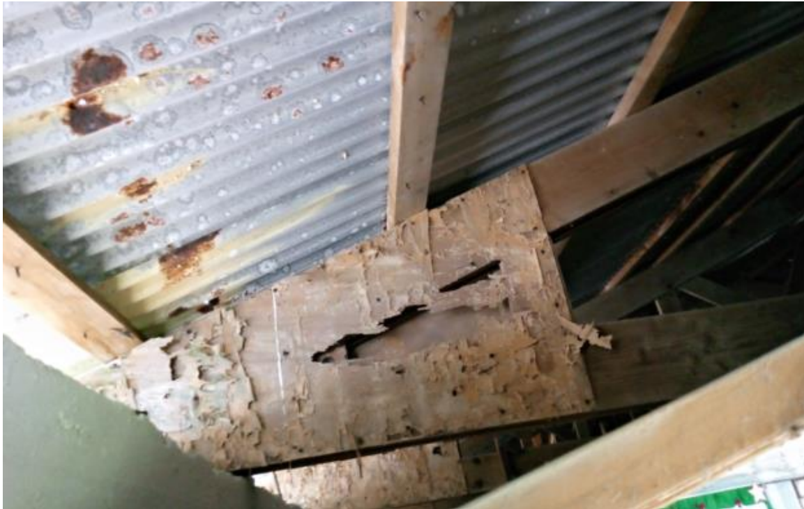
Figure 30. Slightly damaged edge of the Sapota church roof
