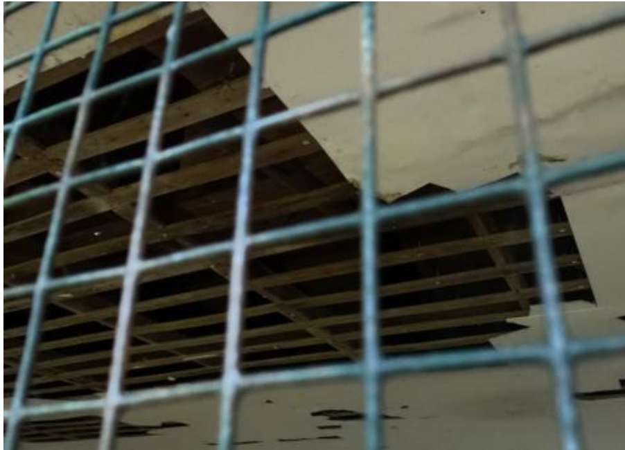
Figure 73. Ceiling of the Mesa elementary school
