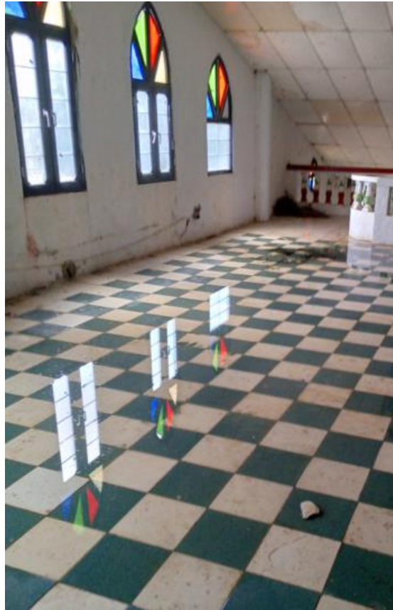
Figure 47. Leaks inside of Fein new church
