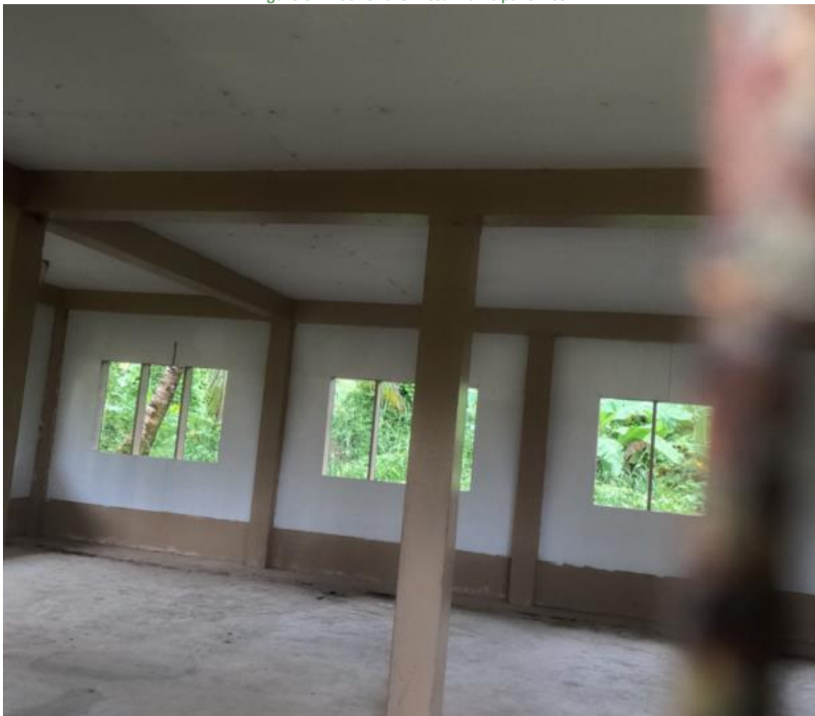
Figure 85. Interior of the Mesa municipal office (solid concrete structure with no leaks)
