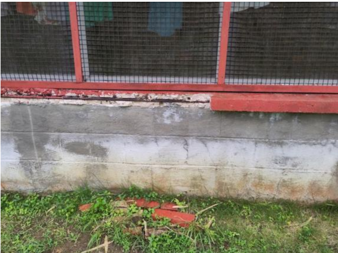
Figure 65. Parish hall damage on outside wall structure.
