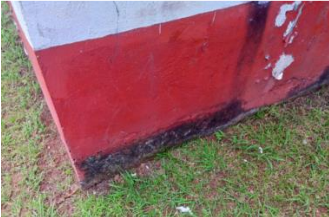
Figure 52. Footings of the Fein new church. no damage, only slightly on the plaster
