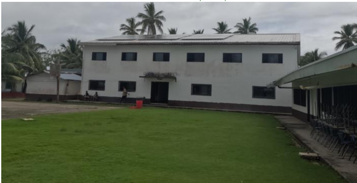
Figure 19. Same view of Sapota 2-storey high school. The concrete blocks on the grass are not connected to a sewage system or tubes.
