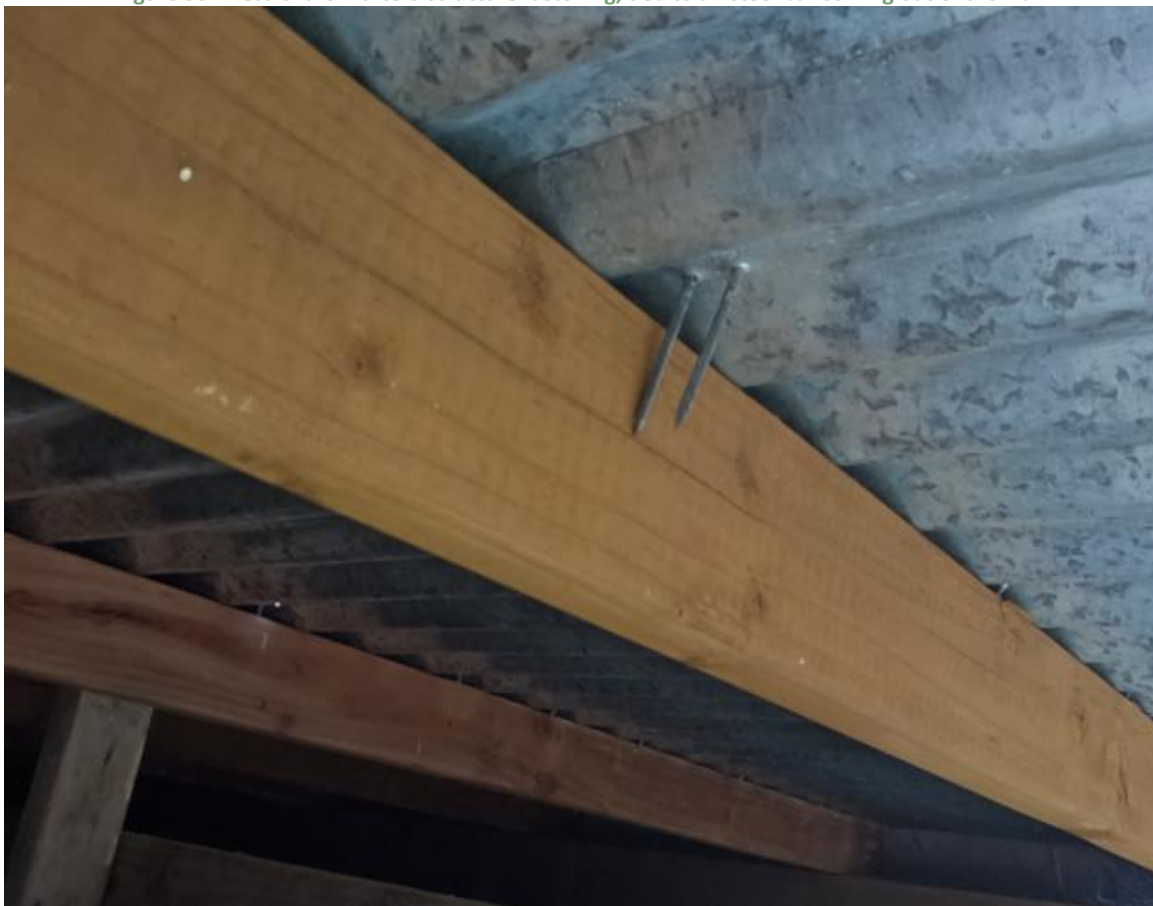
Figure 96. Mesa church roof nails
