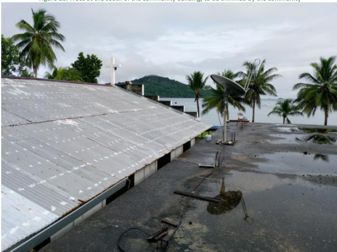
Figure 27. Church and community building (right) roofs, with metal rebars coming out of the structure.
