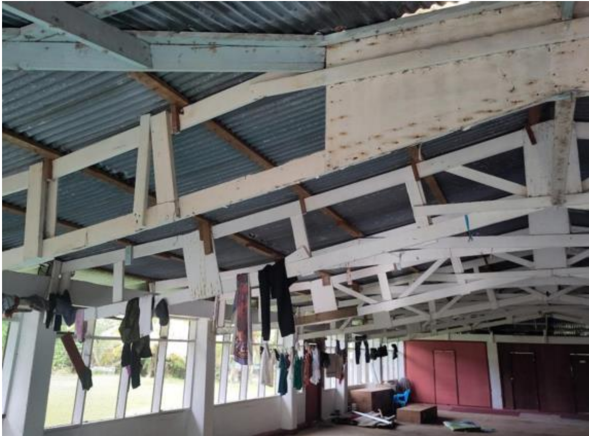
Figure 62. Parish hall damaged wooden structure
