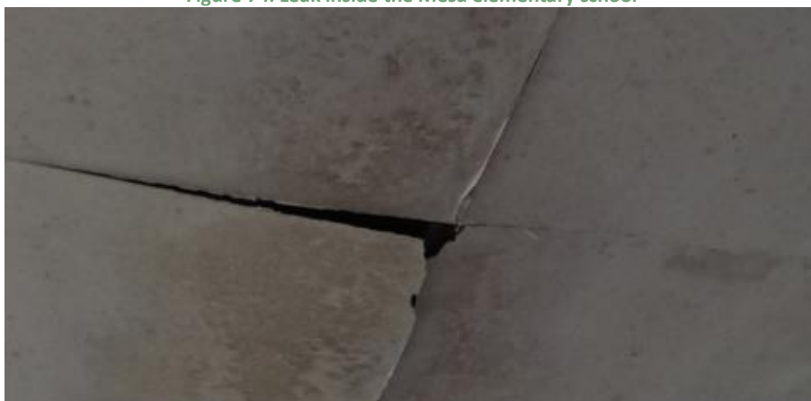
Figure 75. Leak inside the Mesa elementary school 2
