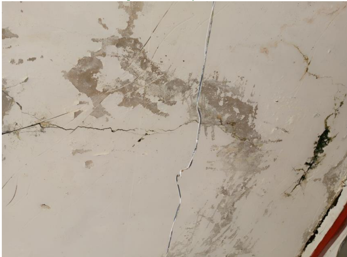
Figure 33. Cracks and humidity on the ceiling of the community building
