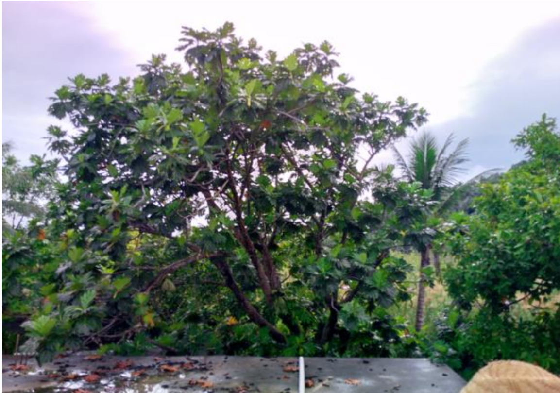
Figure 26. Trees at the south of the community building, to be trimmed by the community
