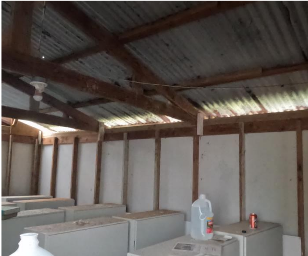
Figure 14. Sapota current technical house for the solar system. It will be emptied such as the small warehouse in order to leave the space for the brand new technical building
