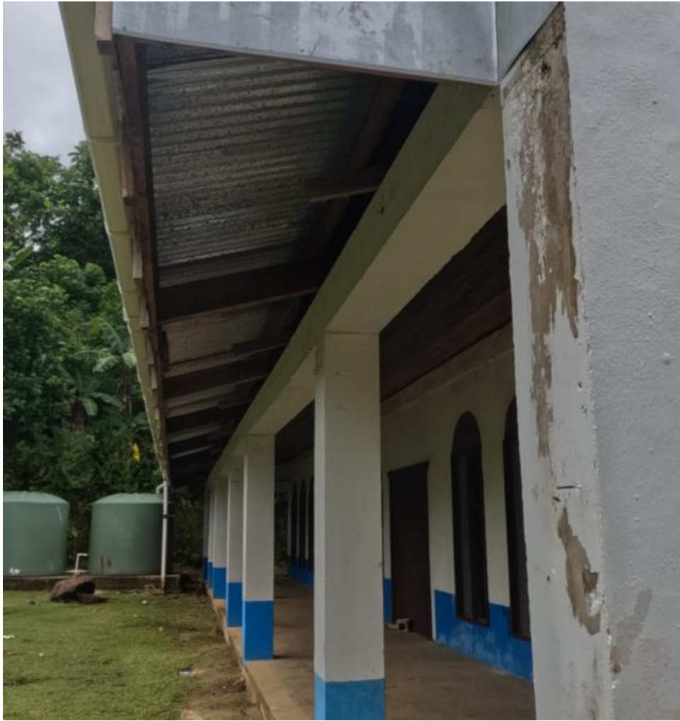
Figure 93. Mesa church side and water tanks
