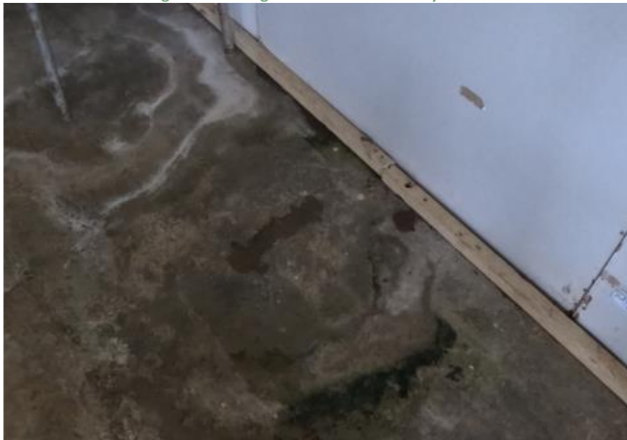
Figure 74. Leak inside the Mesa elementary school
