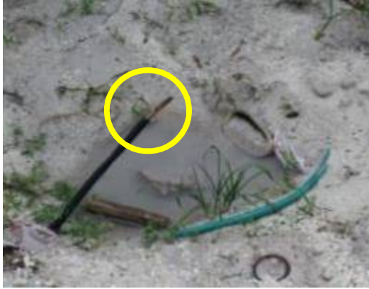
Water accessed at ground level. Pipe blocked off with stick.
