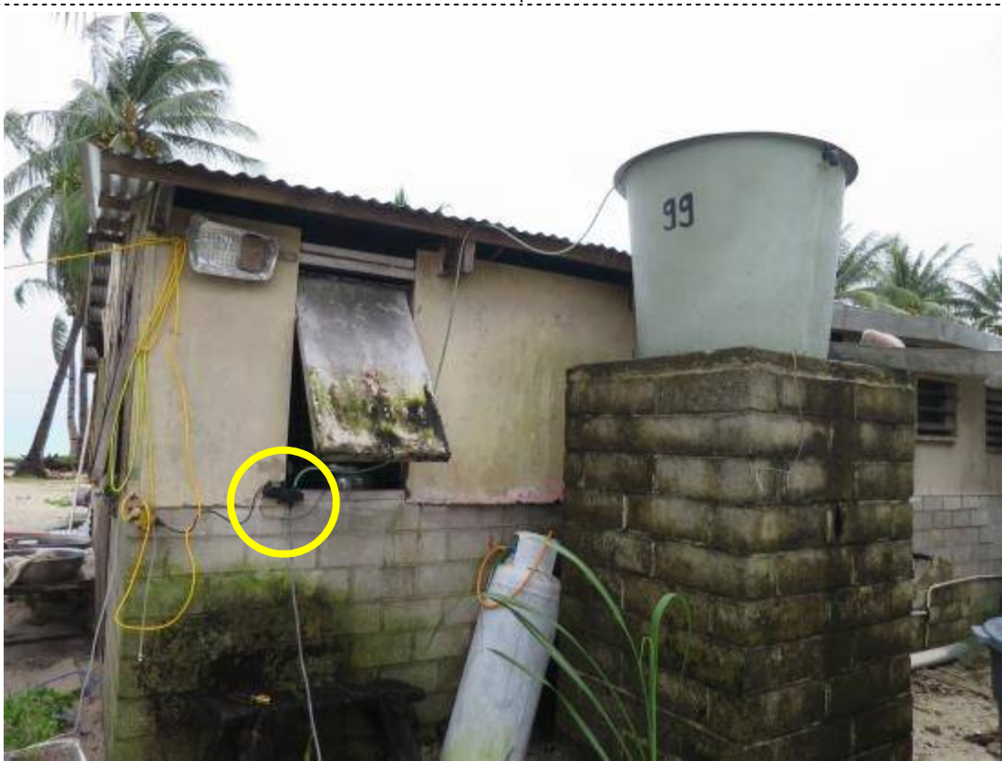
Booster pump at house lifting water into 500 L header tank.
