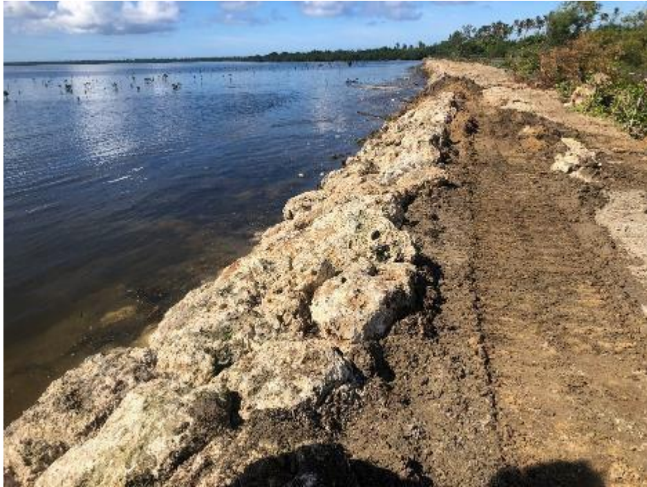
Figure 2-2. The revetment that extends from Ha'atafu to 'Ahau and encloses 2 distinct areas, Kanokupolu wetland in the north, and 'Ahau lagoon in the south. Originally built in the late 1960's, repairs and modifications were carried out in 2014 and 2018; but there are still several areas that require heightening and reinforcing, and the non-return valves along the Kanokupolu section require maintenance.
