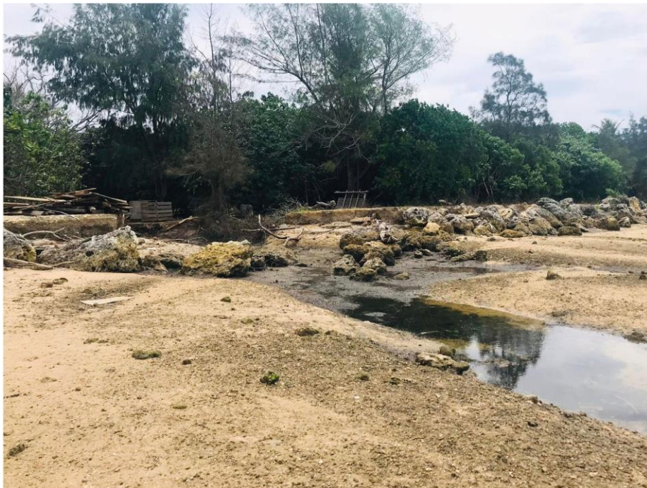
Figure 2-3. One of the blowouts through the coastal track and revetment
