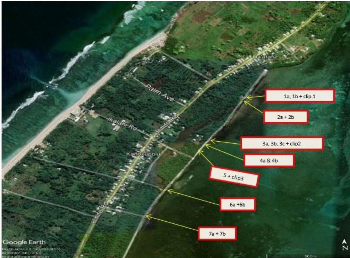
Figure 2-7. Sites of significant damage along the northern 1,350 m of the revetment (Attachment A).
