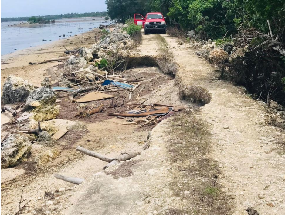
Figure 2-4. Damage revetment and coastal track
