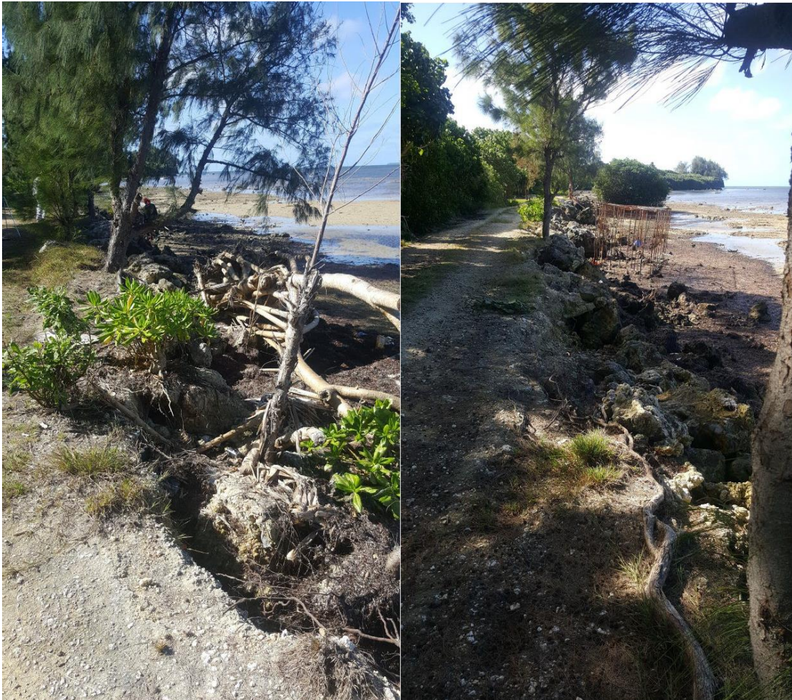
Figure 2-6. Damage to the northern part of the Kanokupolu revetment that occurred during TC Harold.
